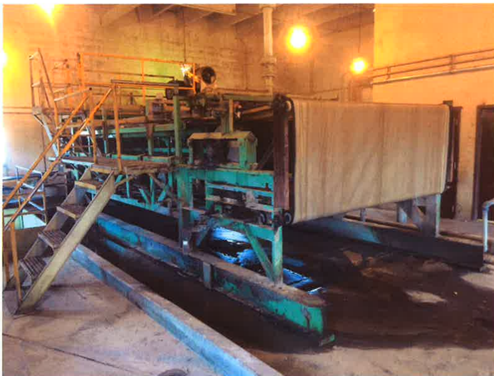
Figure 4-5: Morrow Station Filter Press
