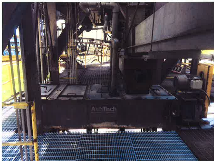
Figure 4-4: Pug mill between steel ash silos and conveyor
