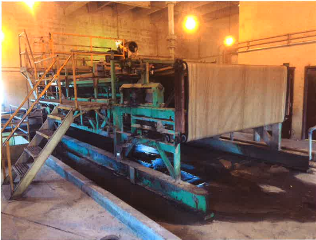
Figure 4-5: Morrow Station Filter Press
